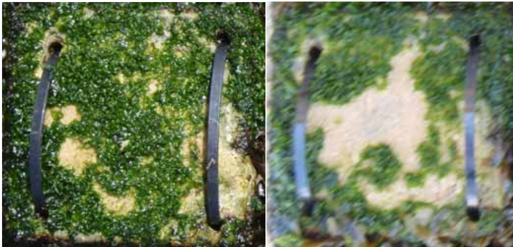
Figure 17. W3 treated tile before water blasting (left) versus the same tile after high pressure water blasting (right).
