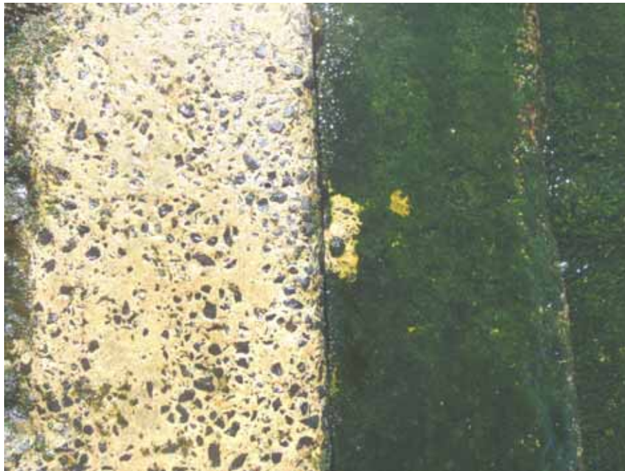
Figure 19. Picture of a step leading into the bay at Clovelly from the southern promenade.
