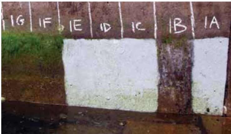
Photo 12 – Malabar Pool Wall
