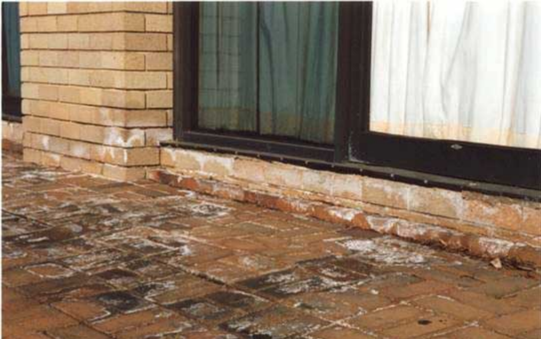
A salt-damaged public building in Western Sydney
