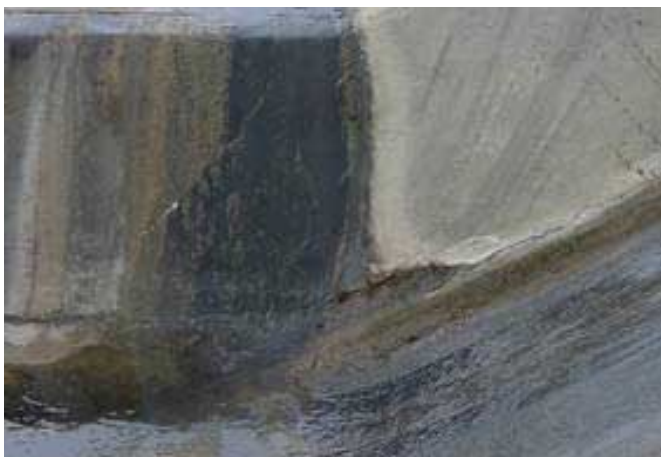
Fig 4: Salt-affected stormwater infrastructure in Western Sydney
